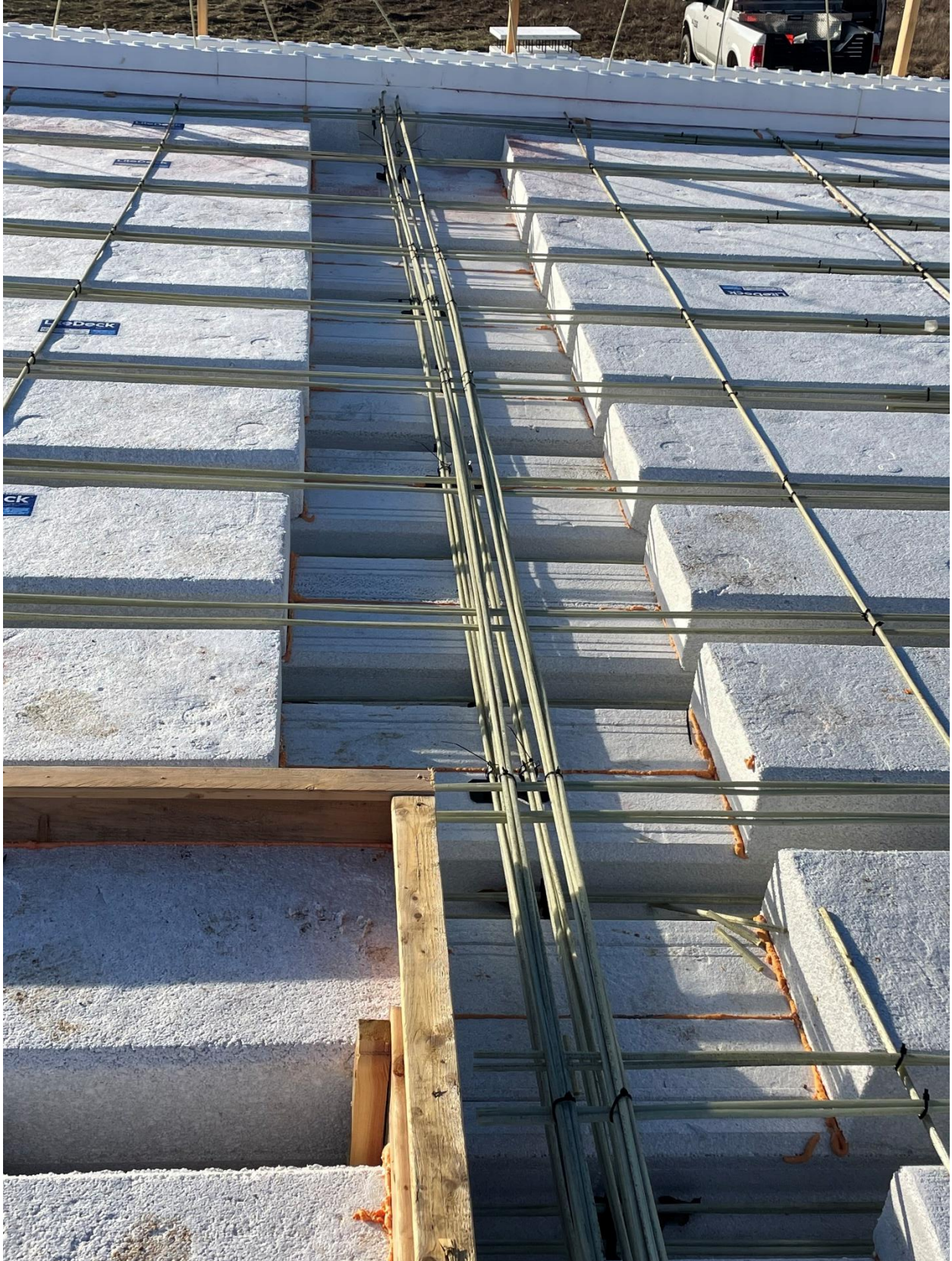
Figure 12 Image showing excessive rebar down main support channel
