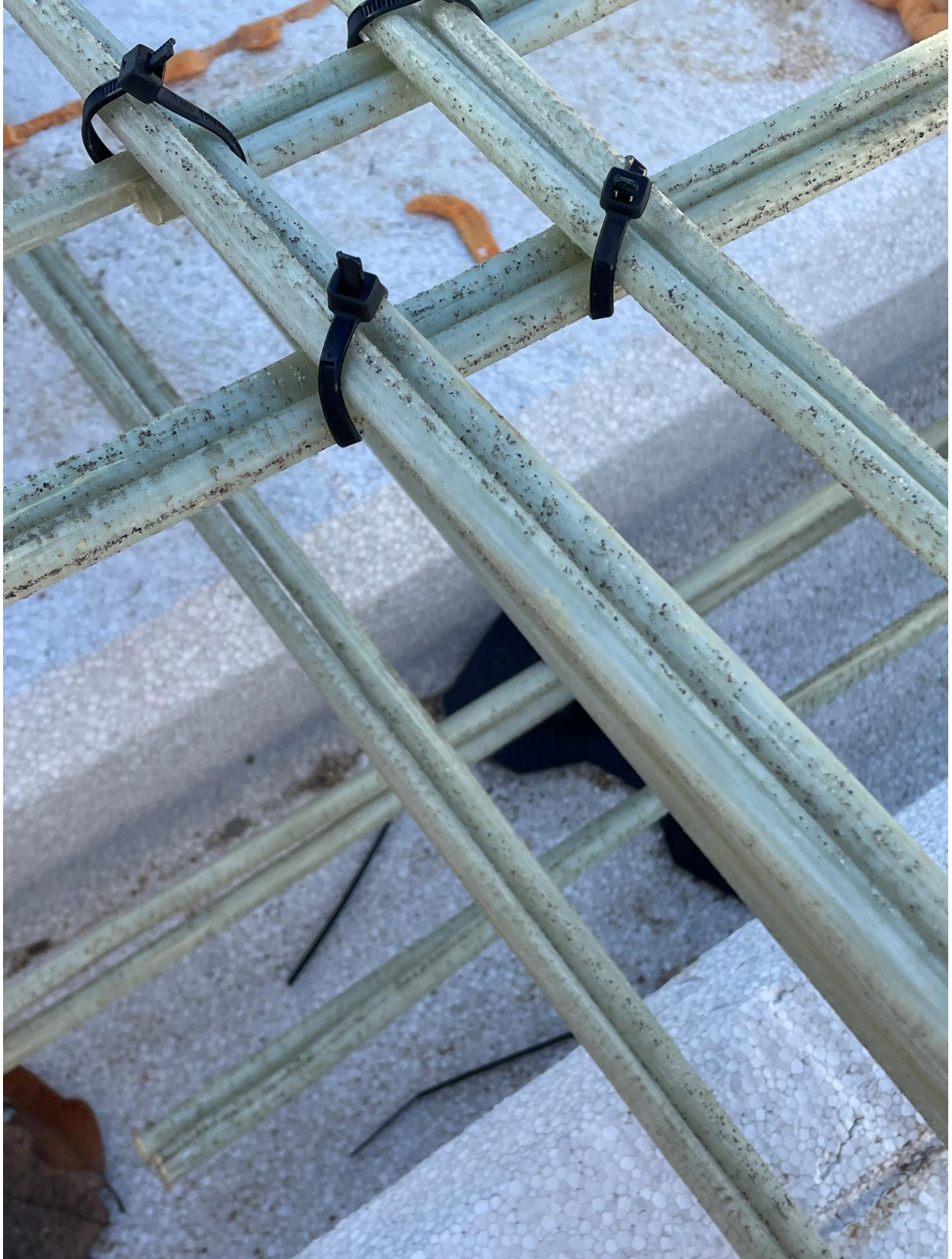
Figure 11 Image showing more rebar than the engineer called for
