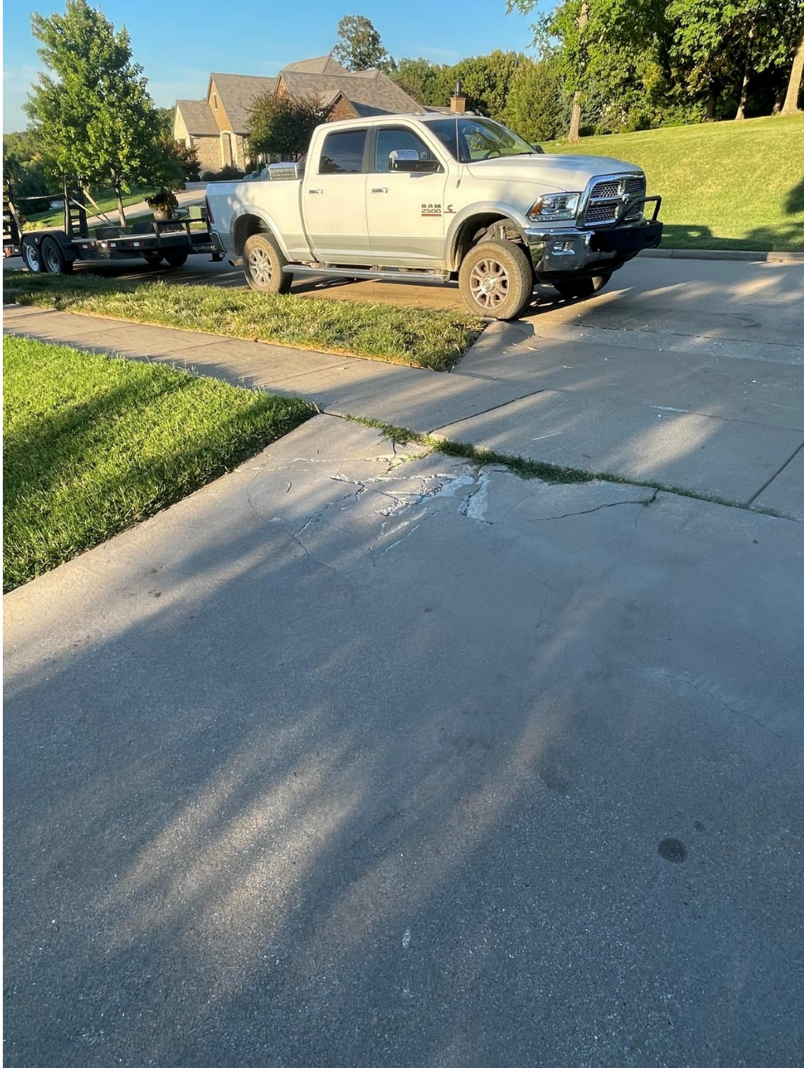
Figure 13 Photo showing cracked concrete. Photo was taken prior to construction. This photo was taken as a precautionary measure just in case the customer accused anyone of damaging the concrete. This shows the customer was willing to lie in her court complaint
