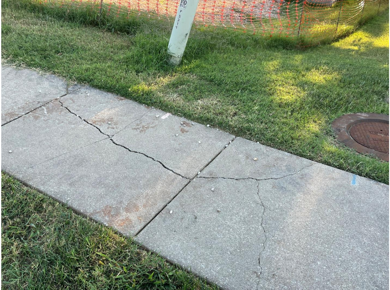
Figure 12 Photo showing cracked concrete. Photo was taken prior to construction. This photo was taken as a precautionary measure just in case the customer accused anyone of damaging the concrete. This shows the customer was willing to lie in her court complaint
