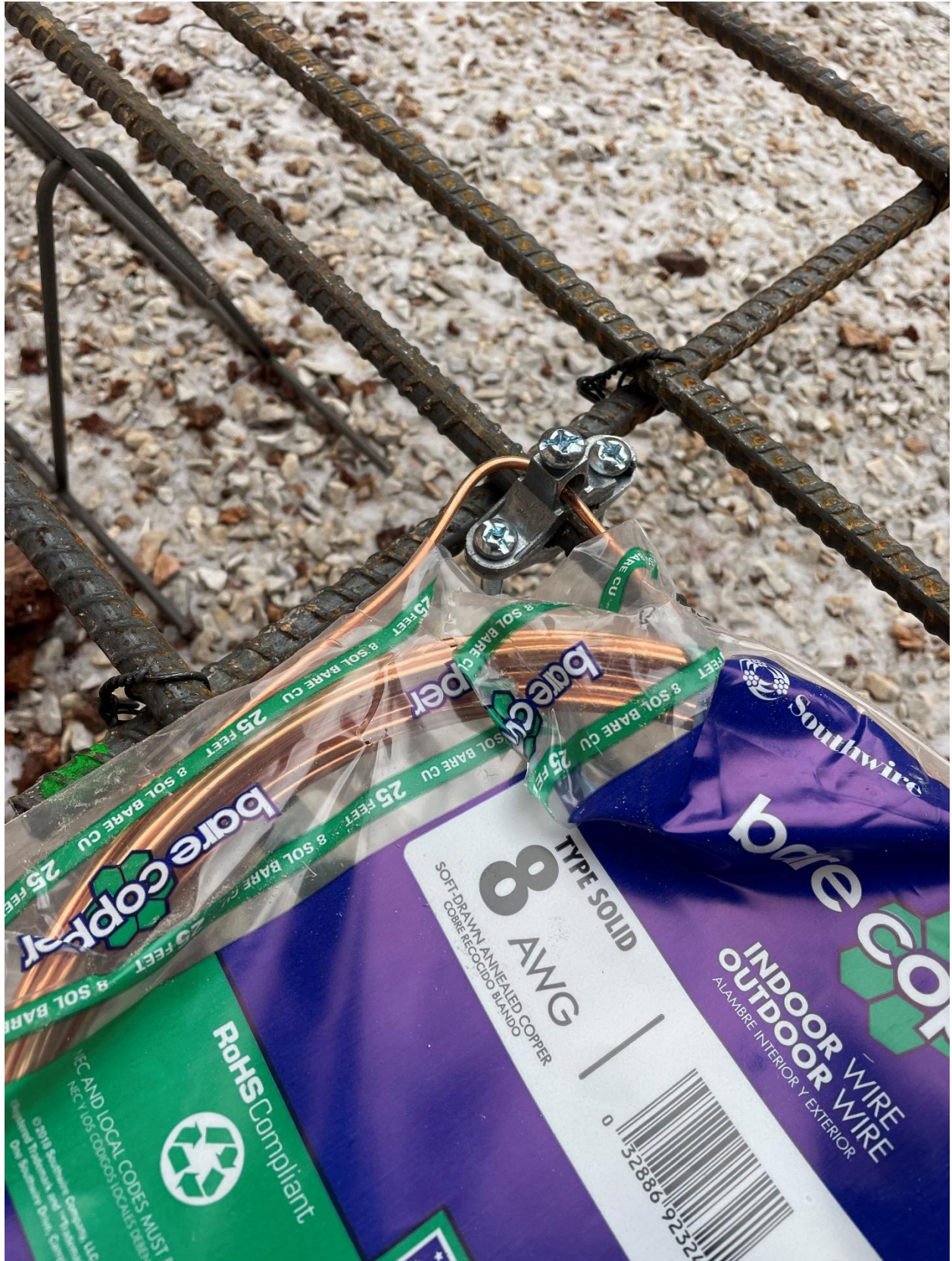
Figure 11 Photo Showing #8 copper bonding wire properly secured to tied rebar
